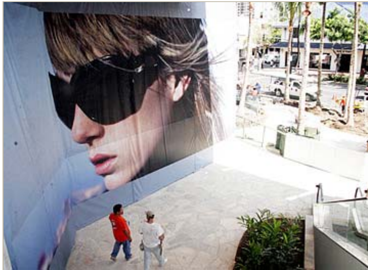
CRAIG T. KOJIMA / CKOJIMA@STARBULLETIN.COM Workmen walk past a large poster for an upscale store at Royal Hawaiian Shopping Center. The center is in the middle of renovation.
