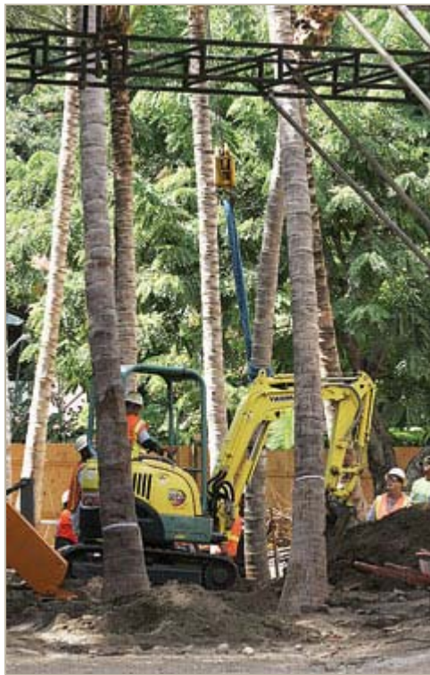
CRAIG T. KOJIMA / CKOJIMA@STARBULLETIN.COM A major overhaul at the Royal Hawaiian Shopping Center included the planting of new coconut trees.
